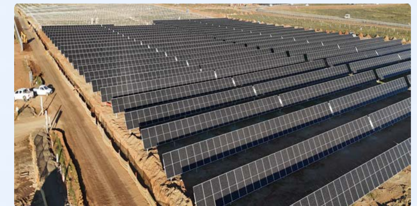
Envusa Energy: Drone view of the solar array project, Koruson 2 cluster, wind and solar project. Partnership between global mining company Anglo American plc and the global leader in renewable energy technology, EDF Renewables, to develop and supply wind and solar energy solutions, at scale, across South Africa.
