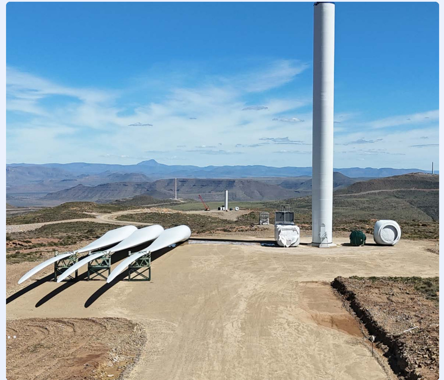
Components delivered to platforms and installation for the Koruson 2 cluster, a wind and solar project by Envusa Energy that will supply renewable energy across the region to Kolomela.
