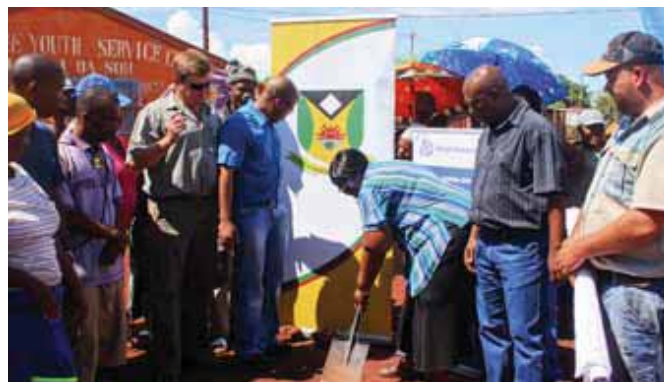
The first SOD turning of this new infrastructure for basic services – from left to right: Petrus Oosthuizen (Consultant MVD Kalahari), Solomzi Henge (previous Technical Director Tsantsabane Municipality), Hazil Mothibi (previous Mayor of Tsantsabane), Gosego Lkgetho (LED Practitioner Kolomela Mine), Dirk Potgieter (contractor Nammic Engineering cc).
