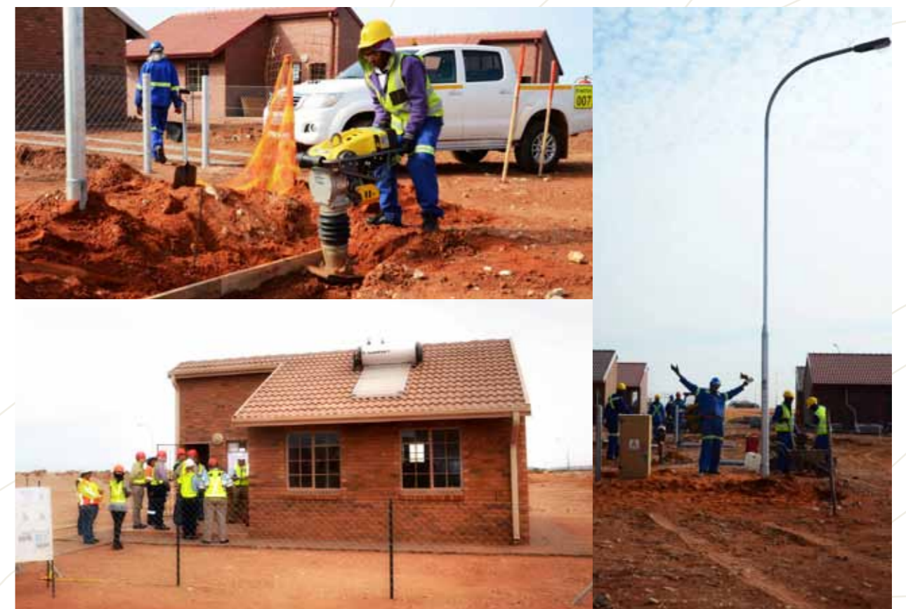
Construction work as part of the Dingleton resettlement was well planned to provide local procurement opportunities to community members.
